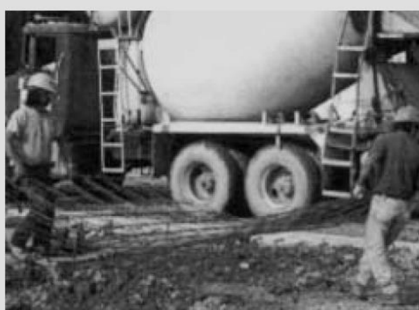
It only takes two workers to easily carry two 8'x 15' sheets of WWR, while rebar requires more expense to tie and place the material.
