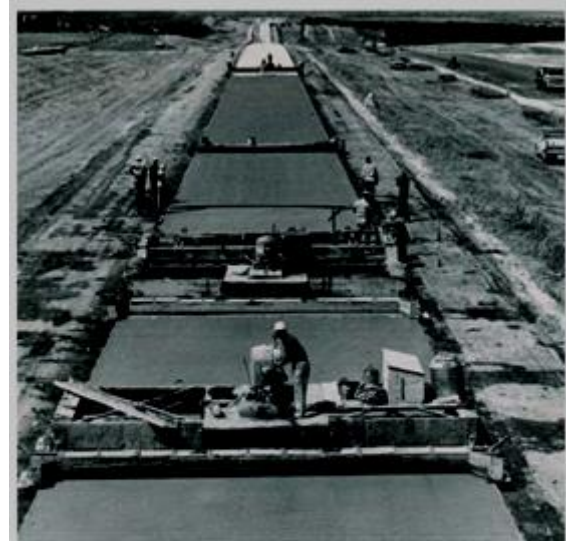
Interstate pavement under construction. This is mesh-dowel pavement going into place on the largest overall highway construction program ever conceived and built in the history of the world.
