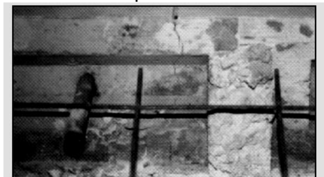
Properly positioned steel below the saw cut control joint allows concrete to crack the full depth and adds load transfer capacity across the joint.
